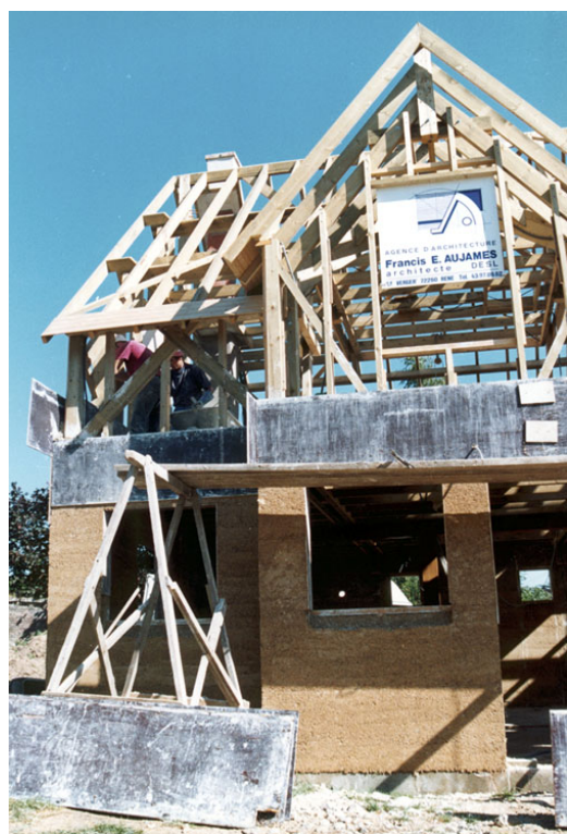
Fig. 24. New building in France being constructed entirely of hemp. Wall castings are a conglomerate of Isochanvre® lime-hemp, for production of a 200 mm thick monolithic wall without an interior wall lining. (Courtesy of M. Périer, Chènovotte Habitat, France.)
