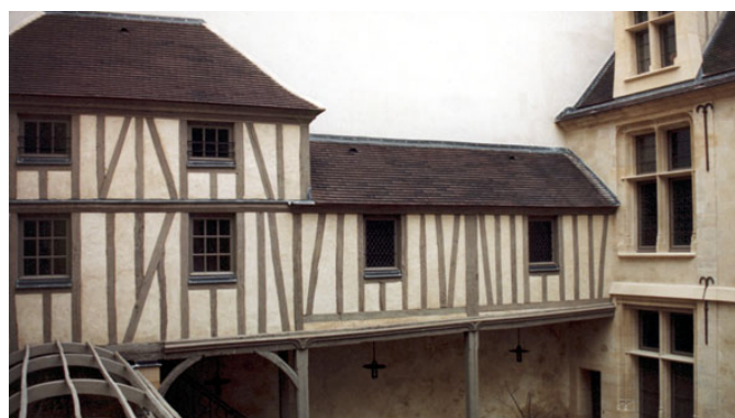
Fig. 26. Renovation of plaster walls of a traditional timber frame 16 th century house (Mansion Raoul de la Faye, Paris) with Isochanvre® lime-hemp conglomerate. (Courtesy of M. Périer, Chènovotte Habitat, France.)
