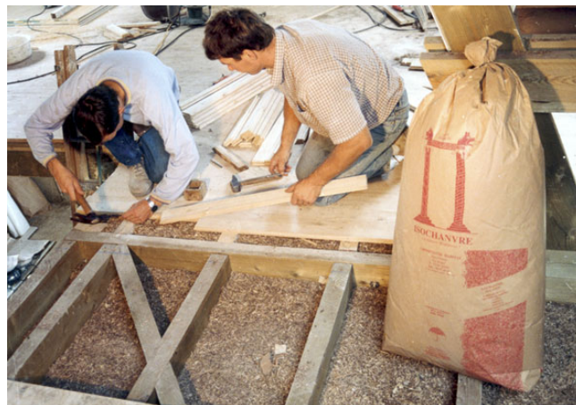
Fig. 21. Loose Isochanvre® thermal insulation being placed between joists. (Courtesy of M. Périer, Chènovotte Habitat, France.)
