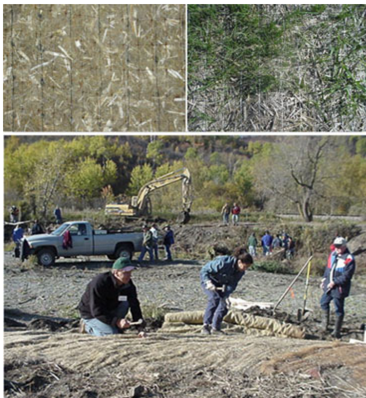
Fig. 32. Hemp-based erosion control blanket. Top left: Close-up of 100% hemp fiber blanket. Top right: Grass growing through blanket. Bottom: Demonstration of installation of blanket, near La Rivière, Manitoba. (Courtesy of Mark Myrowich, ErosionControlBlanket.com)
