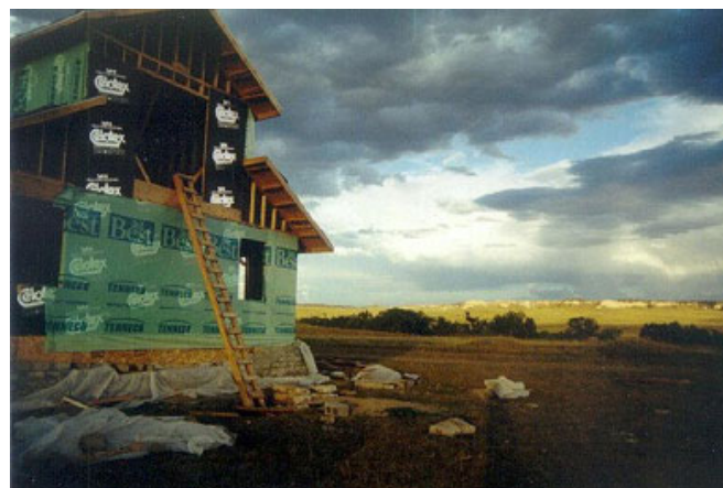
Fig. 25. The “hemp house” under construction on the Oglala Lakota Nation (Pine Ridge Reservation), South Dakota. Foundation blocks for the house are made with hemp fiber as a binder in cement. Stucco is also of hemp. Shingles are 60% hemp in a synthetic polymer. Hemp insulation is used throughout. (Courtesy of Oglala Sioux Tribe, Slim Butte Land Use Association, and S. Sauser.)
